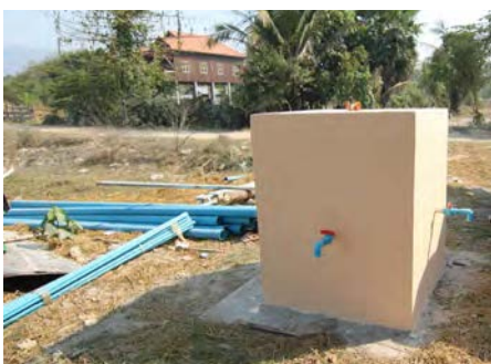
Water point connection
